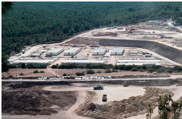
Figure 7. The construction of the new camp in Vastria. Photo credit: Davide Marchesi.
