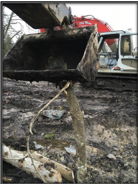
FIGURE 22. COTTONWOOD STAKES ARE BEING INSERTED BY THE EXCAVATOR BUCKET EXERTING GENTLE PRESURE.
