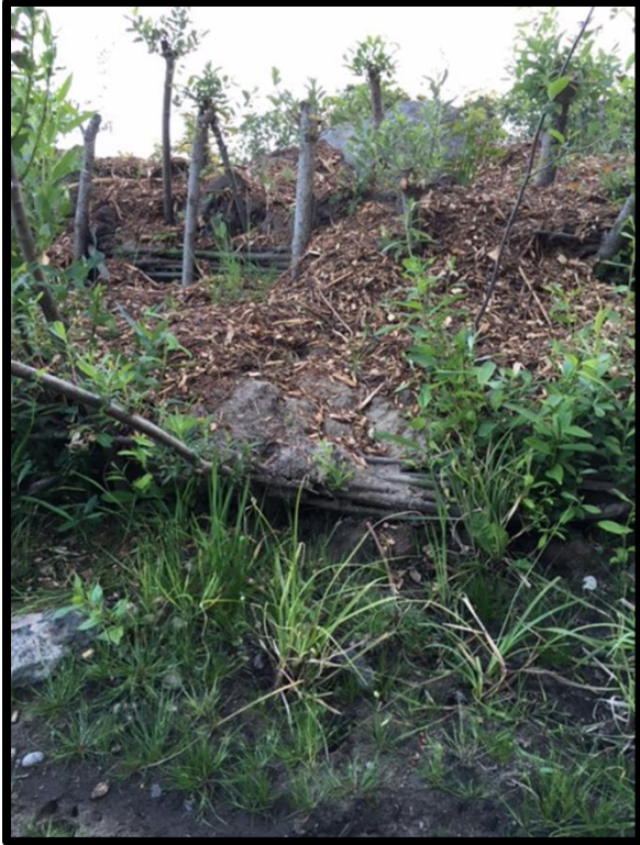
FIGURE 28. WILLOWS HAVE LEAFED OUT AROUND THE DAMAGE FROM OOZING WET CLAY.
