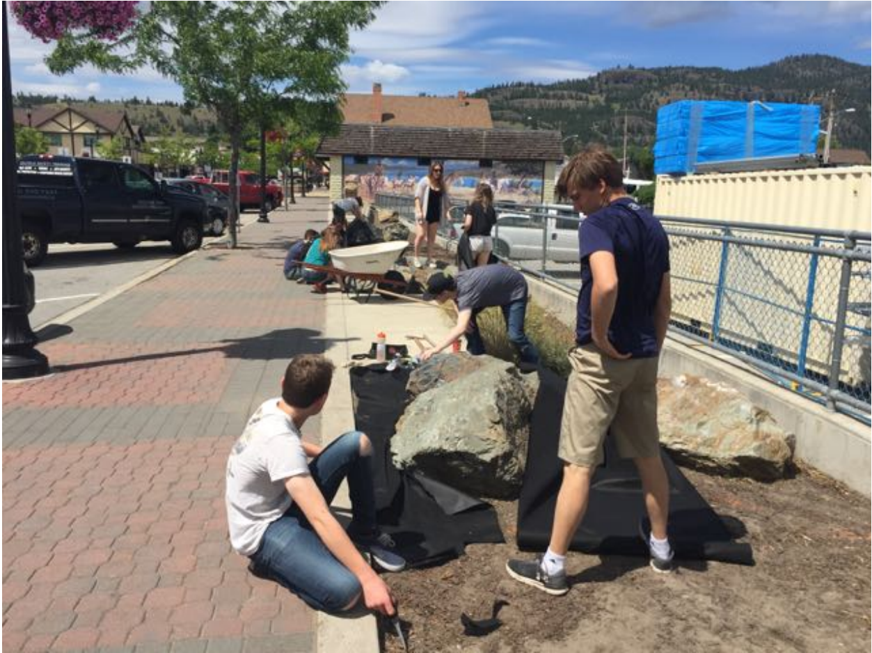
Figure 8. Pulling out the last of the weeds & laying down landscape fabric (Image Source: Tanya Brouwers)
