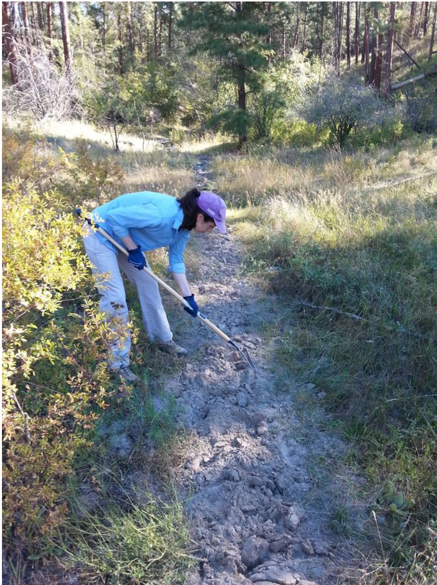
Figure 12. Decompaction of trail tread. The trail tread was manually decompacted by digging followed by raking to break-up large clods. (Photo: T. Redding)
