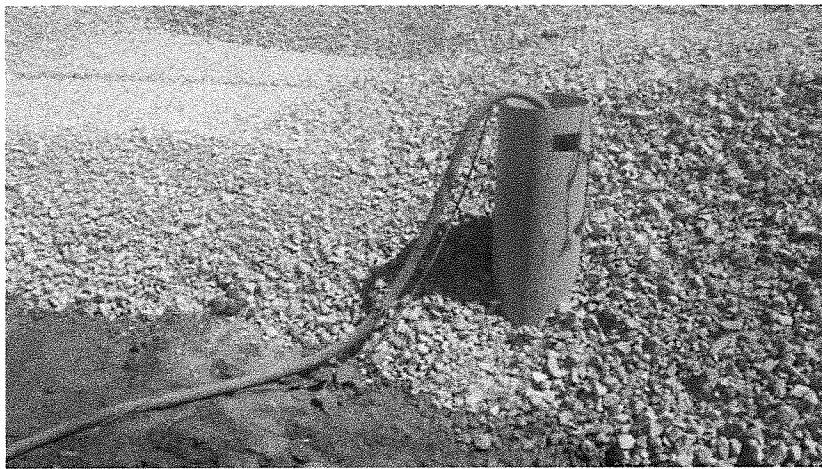
Figure 7: A Sump with a 3" Pump inserted
