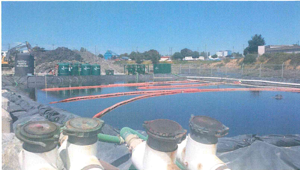
Figure 8: Settling pond and water treatment system in background
