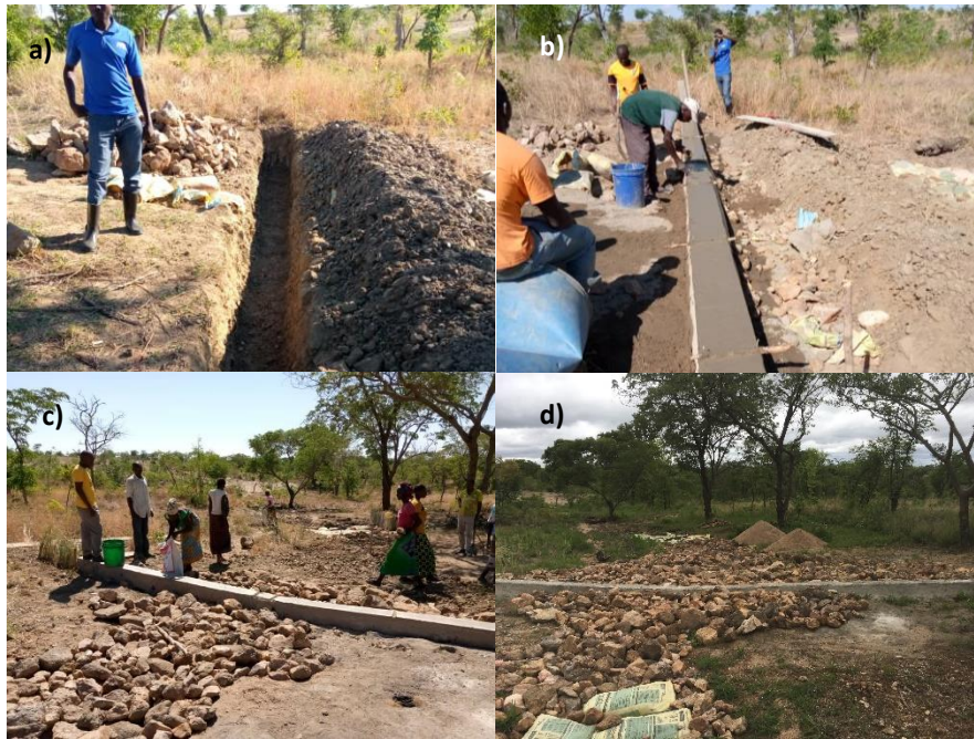
Figure 8: a) Flood-spreading sill trench; b) levelling top of sill; c) constructed sill above gradient drop; d) finished sill after rock placement
