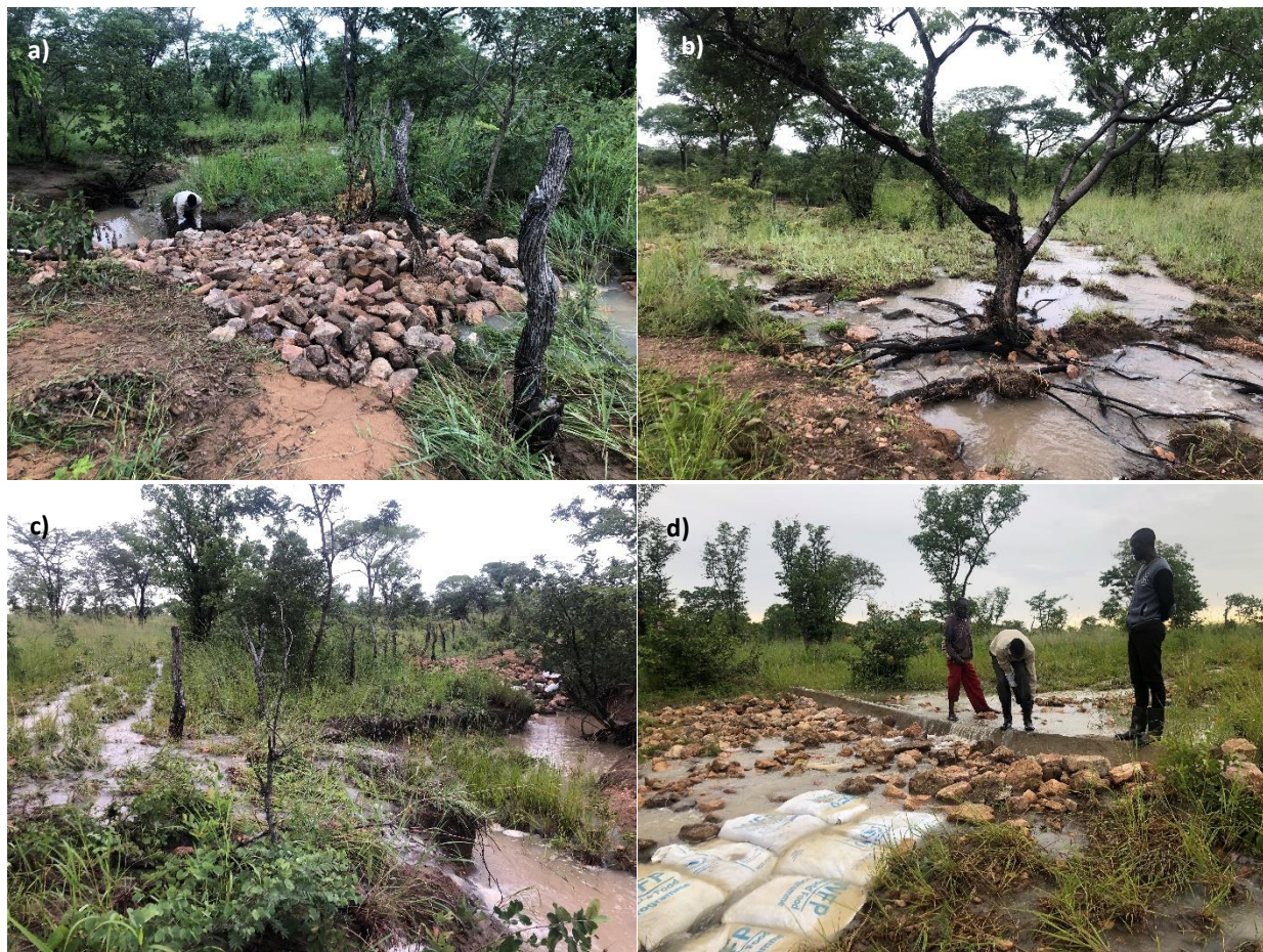
Figure 15: a) Plugged gully at outlet of dam spillway; b) flat area of new erosion on unprotected land; c) overflow re-routing flowing over unprotected gully head; d) flood-spreading sill
