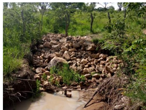
Figure 11: Plugged gully on dam spillway the
