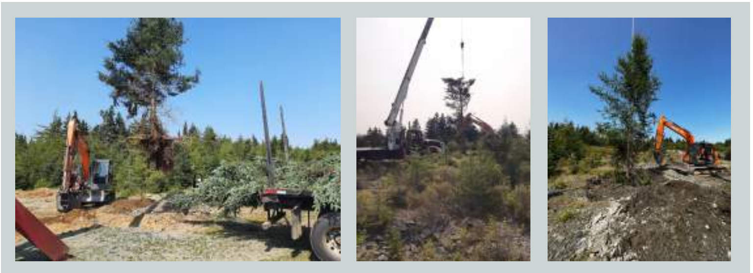
Figure 7 - Heavy machinery was used for snag installation, including a truck to transport trees to the site, an excavator to dig holes in the rocky substrate, and a crane to lift the trees into the holes. Photos by Aaron Dowding
