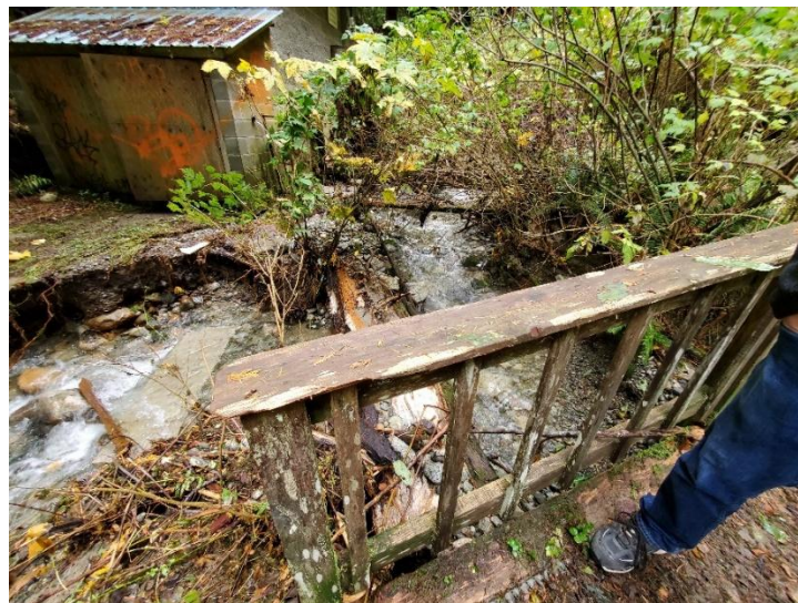
Figure 1: Photo showing undercutting of bank near SCRDR well pumphouse (SCRDR, 2021)
