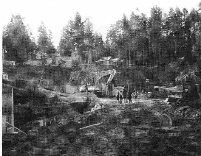
Poets Cove February 10, 2003. View of construction site for Poets Cove Resort and Spa (Photo courtesy of E. McLay).
