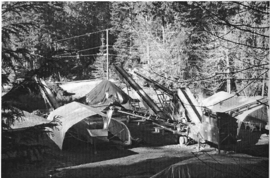
Mechanical Gravel Sorter imported to Poets Cove to expediently sort Ancient Human Remains and Artifacts from Construction Backfill, February 2005 (HTG).
