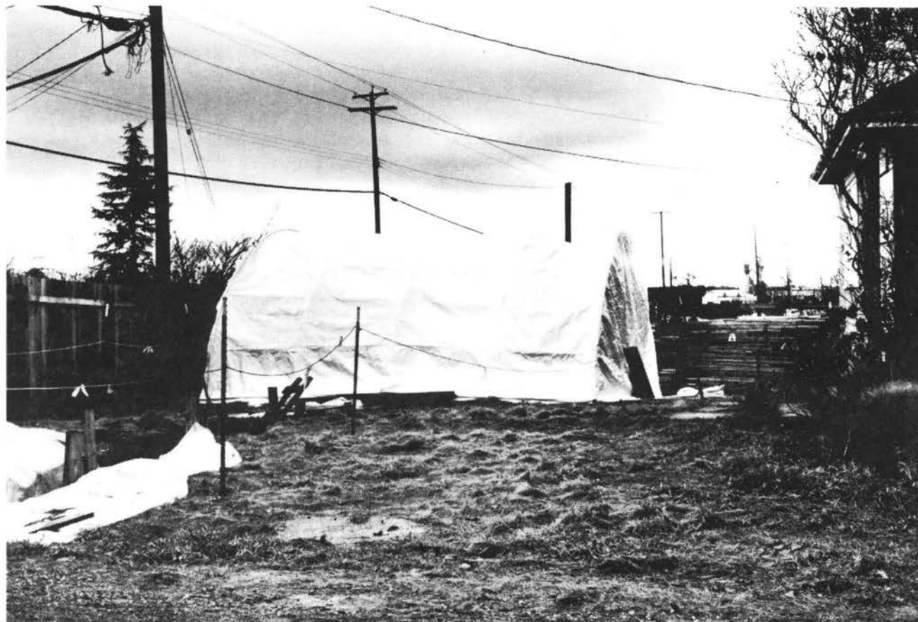
GREENHOUSE EFFECT: Plastic roof over excavation area at St.Mungo Cannery site is the only way workers can shelter from miserable weather, as they continue to dig throughout the winter. Old house at right is used as site office & lab.
